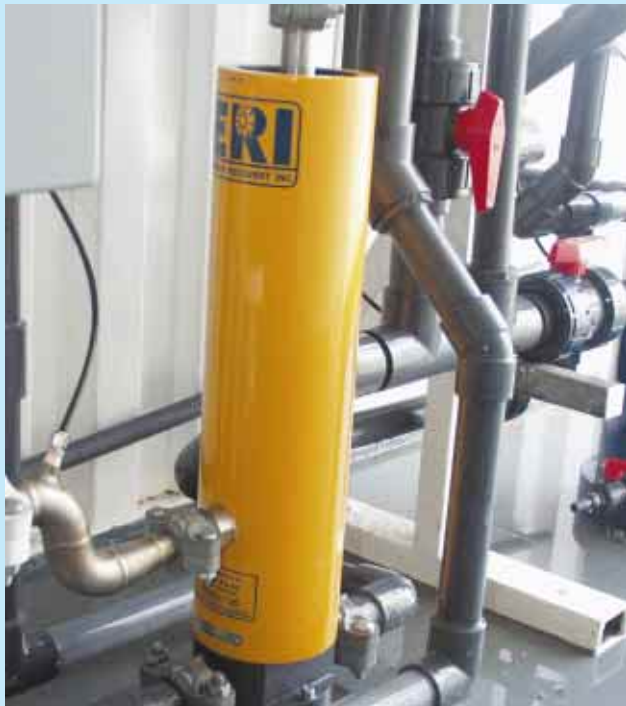
The PX exchanger in the pilot plant
